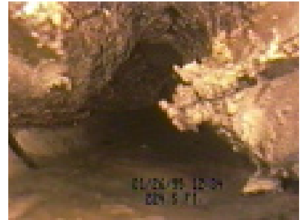
Above: Fat, oil and grease are beginning to accumulate in a sewer and restrict the flow of wastewater. This picture was taken with a special videocamera we use to inspect the sewer system.
