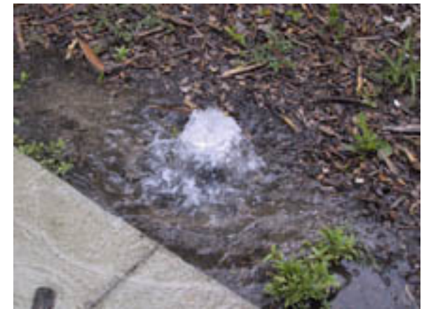
A BROKEN SPRINKLER HEAD CAN WASTE MUCH MORE WATER THAN A LEAKING FAUCET.
