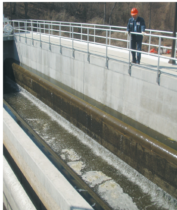
Right: One of the new filters at our Mason Farm Waste- water Treat- ment Plant.
