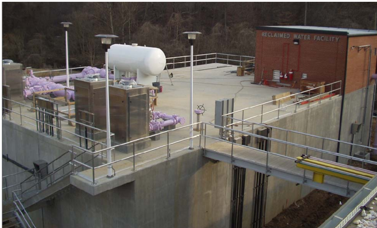
The Reclaimed Water Pump Station at our Mason Farm Wastewater Treatment Plant. Reclaimed water pipes are painted or wrapped in purple to distinguish them from water and sewer lines.
