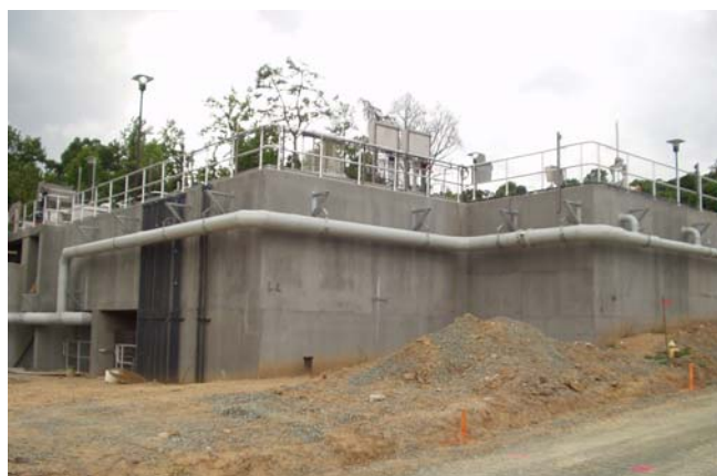
The new enclosed headworks at our Mason Farm Wastewater Treatment Plant eliminated a significant odor source.
