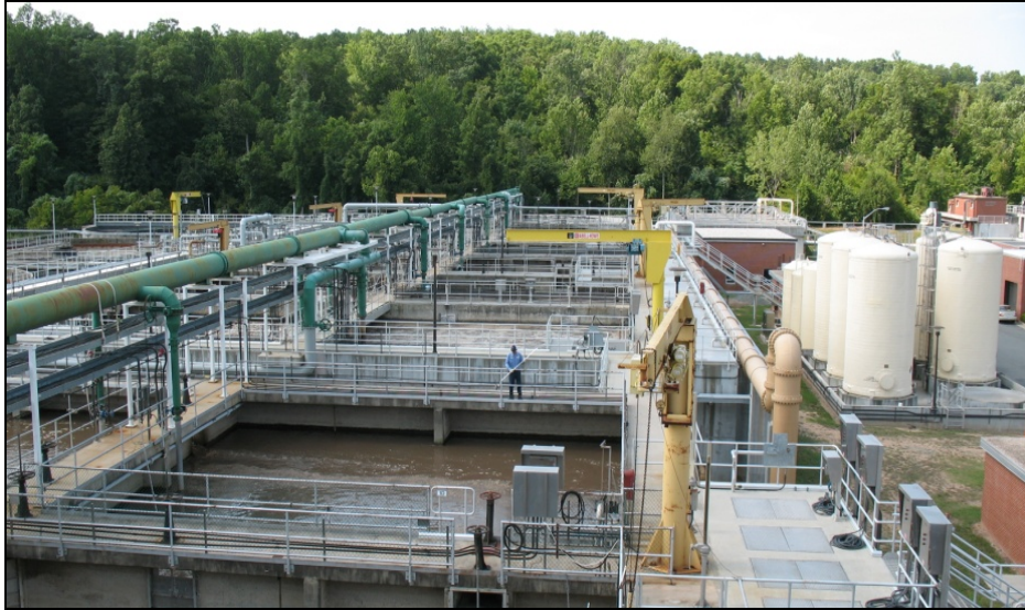
OWASA Operator checking the aeration basin at Mason Farm WWTP
