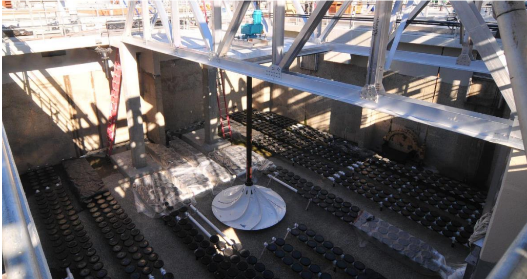
Work to install energy and chemical efficient equipment in the aeration basins at OWASA's Mason Farm Wastewater Treatment Plant
