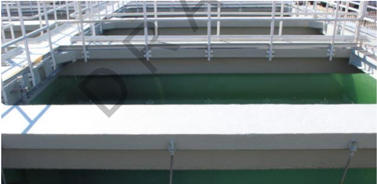
Clarification Tanks at the Jones Ferry Road Water Treatment Plant
